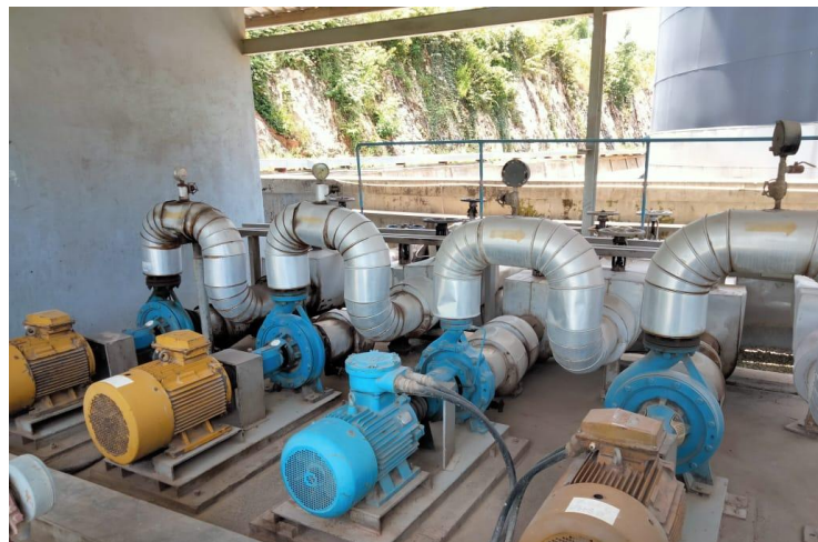
LSB Pump Stations
