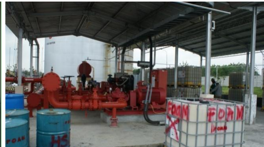
Fire Protection System
