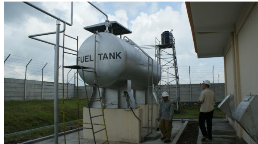
Fuel Tank For Power House
