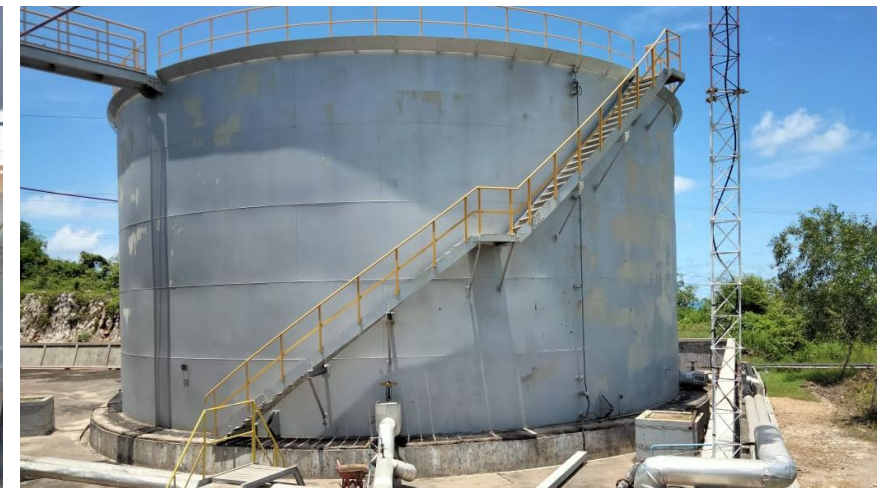
HSD Tank Storage at LSB Port
